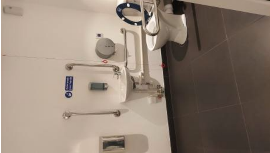
The accessible toilet. Showing the handrails, lowered sink and hand dryer and pull cord.
