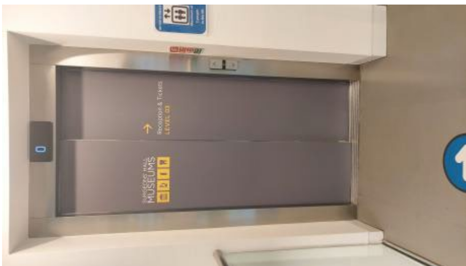
Photo showing the lift door
